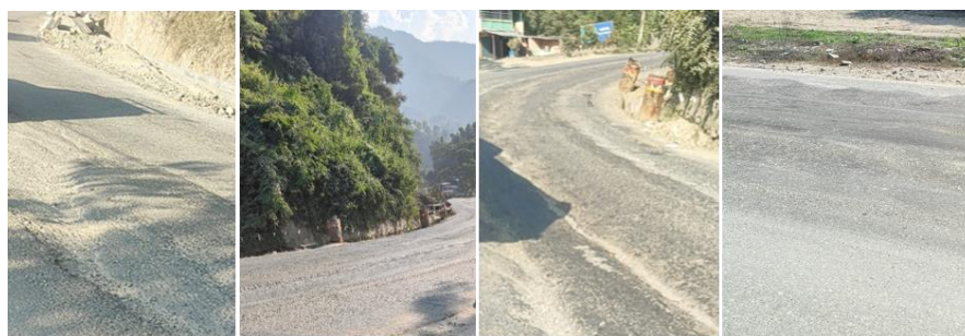
Figure 2: Rutted and depressed road surfaces in the heavily loaded truck lane of Prithvi Highway: Piplamod, Kathmandu (First Figure), Galchi Height, Dhading (Second Figure), Richoktar, Malekhu, Dhading (Third Figure), and Bishaltar, Chitwan (Fourth Figure)
