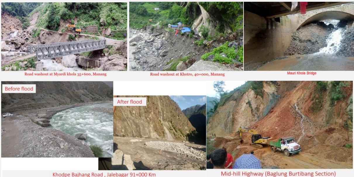
Figure 7: Representative evidence of Highway Infrastructure damage due to flood, landslide, and river toe cut resulting from extreme precipitation.
